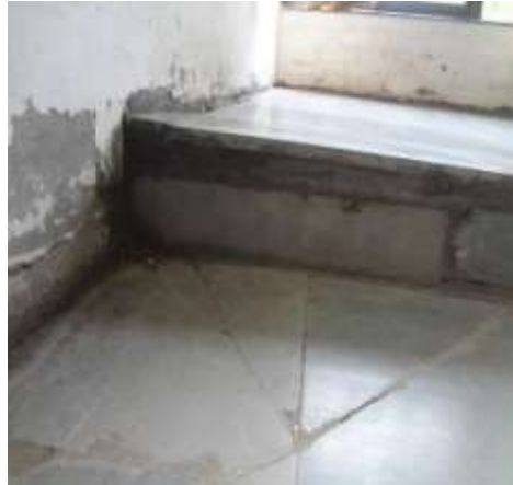
Photograph 9: Flooring/ Improper leveling
