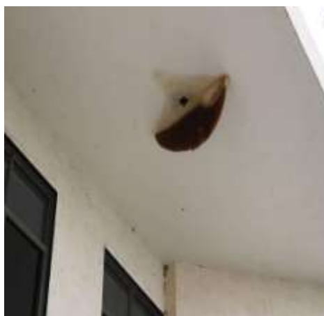
Photograph12: Lack of maintenance
