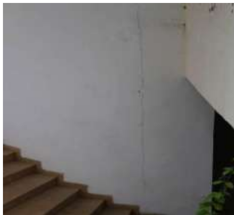
Photograph 10: Beam-wall/Vertical crack(Expansion joint)
