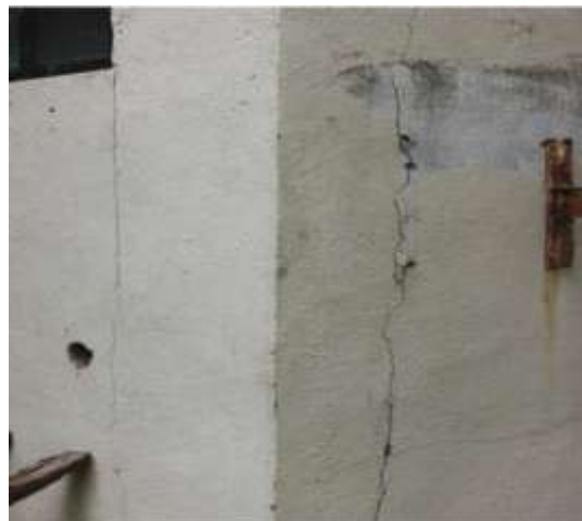
Photograph 2: Vertical crack (Wide crack)Due to Thermal stress
