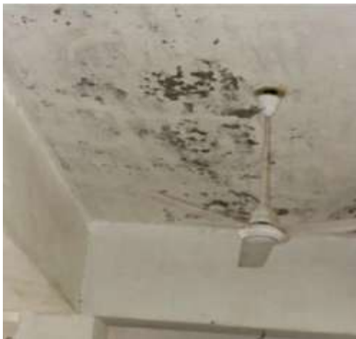
Photograph 4: Leakage and Dampness
