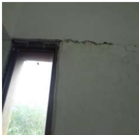
Photograph 11: Beam-wall (Horizontal crack)
