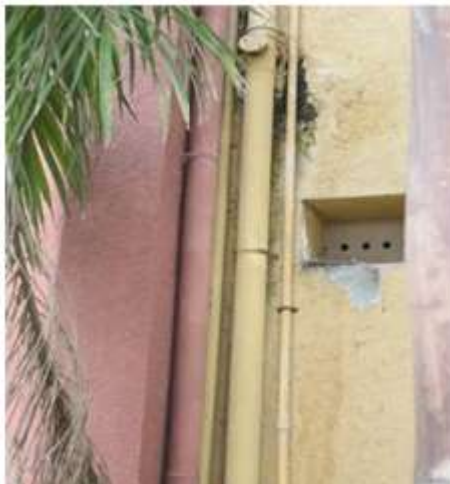
Photograph 5: - Improper/poor drainage pipe
