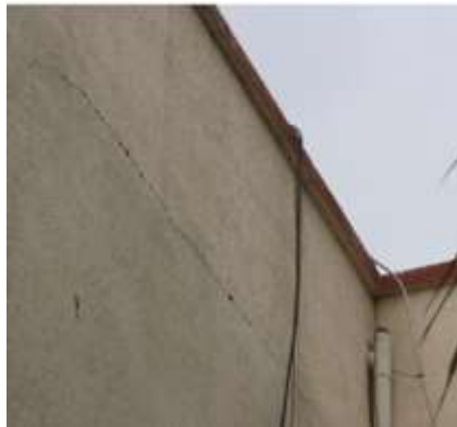
Photograph6: Horizontal crack due to shrinkage
