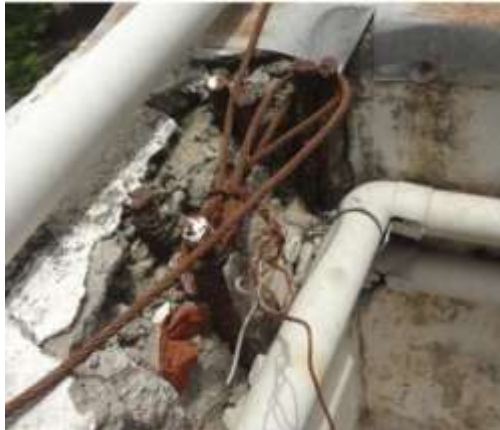
Photograph 3: Open reinforcement and Environmental Effect
